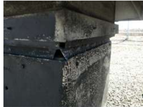
Improper Seating of Housing
