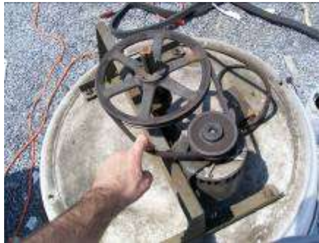
Loose or Broken Belts
