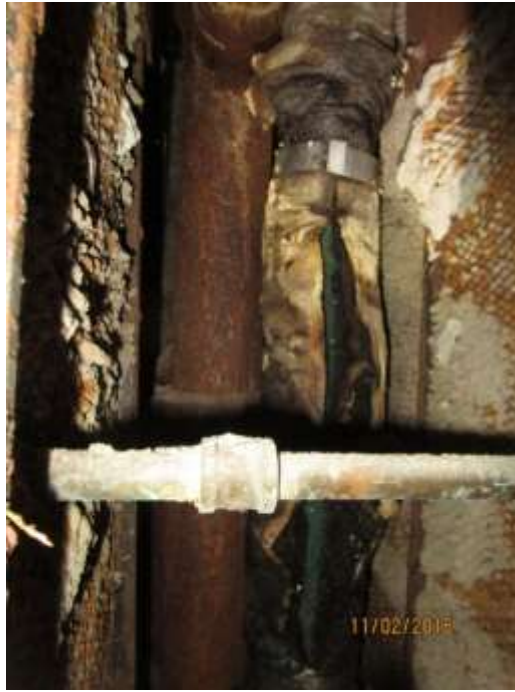
Damaged insulation on cold water riser
