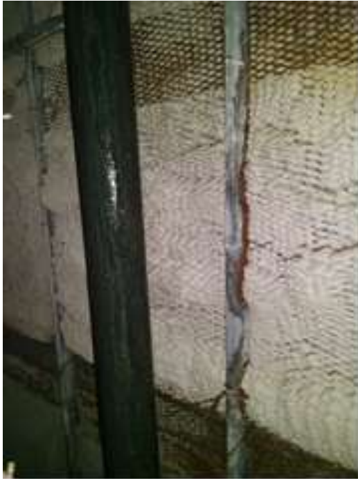
Missing insulation on cold water riser
