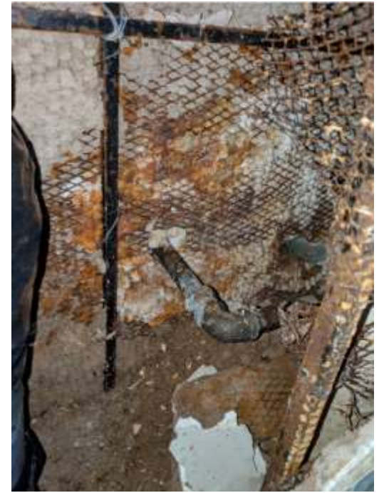
Missing insulation on cold water supply t
